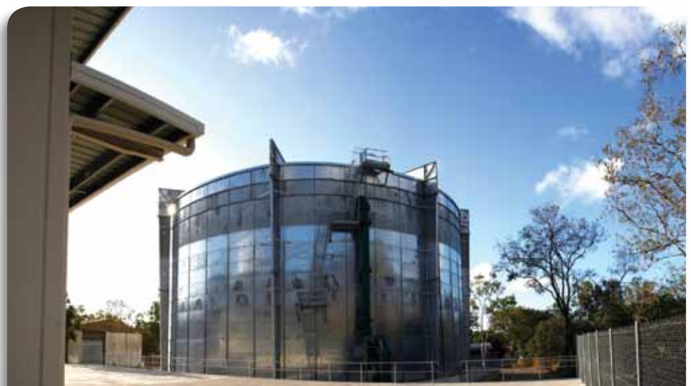
JCU Water storage for the central district cooling system.
