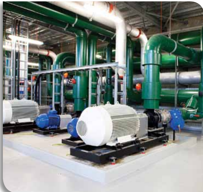
JCU chiller plant room
